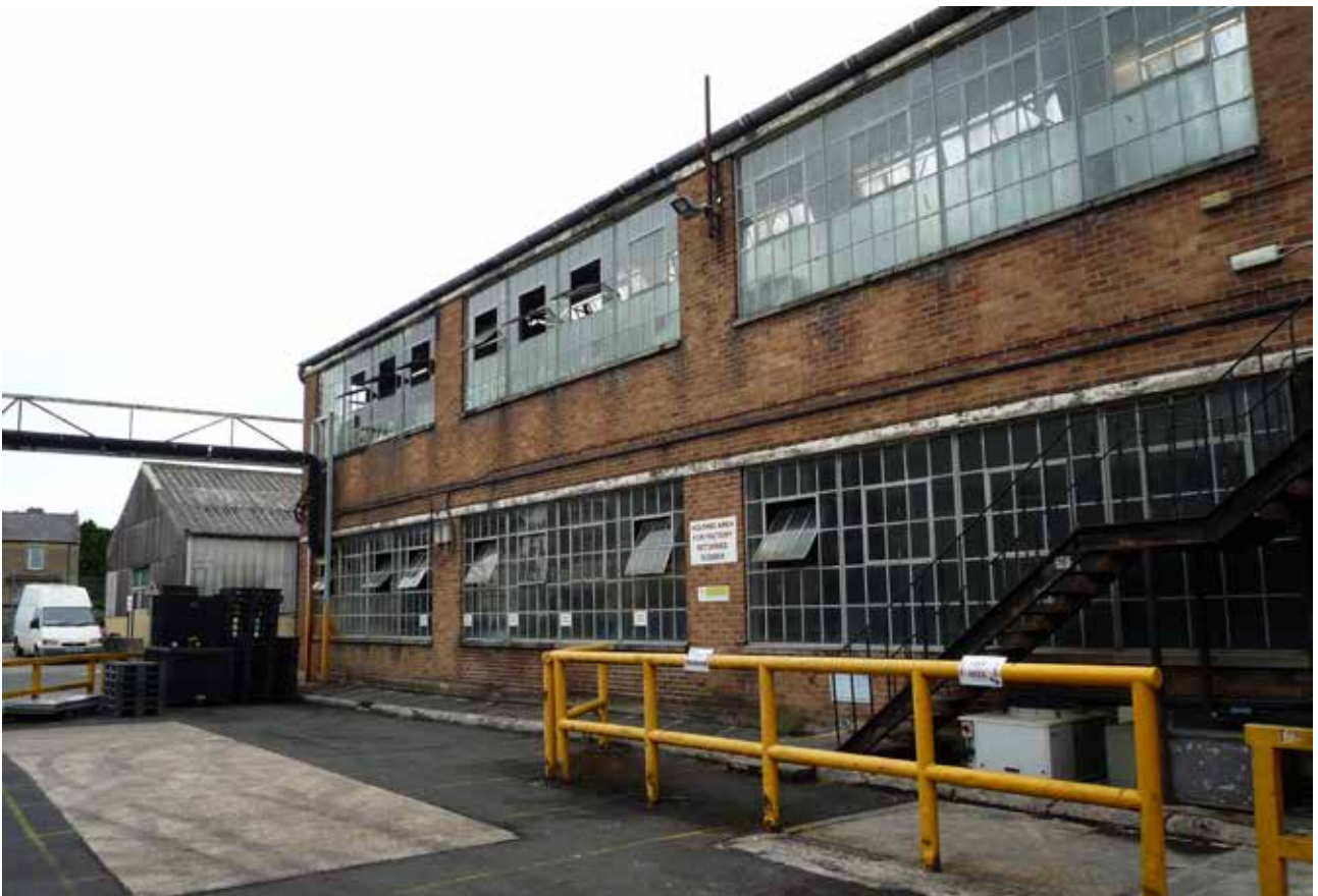
3.21 Main Production Hall
