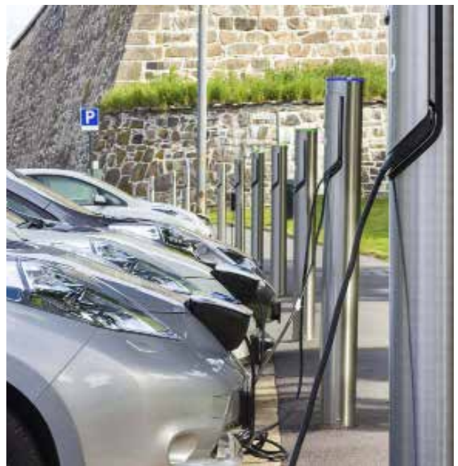
Figure 56: Electric charging points
