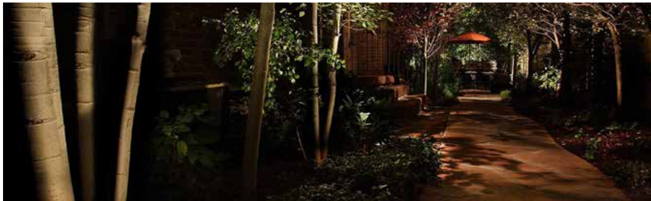
Figure 199: Example of down lighting which was used to illuminate the pathway.
