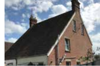
Figure 53: Red brick with cat-slided rear roof at the rear and dark clay pantiles.
