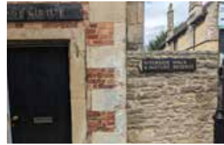
Figure 35: Stone quoin corner and brick detailing of building adjacent to stone boundary wall.
