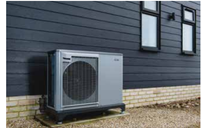
Figure 153: Example of an electric heat pump that is placed to the back of the house, whilst its grey colour fits nicely with the black weatherboarding of the property.
