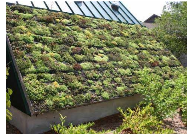
Figure 156: Orientate green roofs and walls to optimal sunlight radiation and minimise the effect of overshadowing
