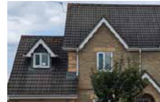
Figure 55: Dark clay pantile roof with dormers and quoin detailing at the corner.
